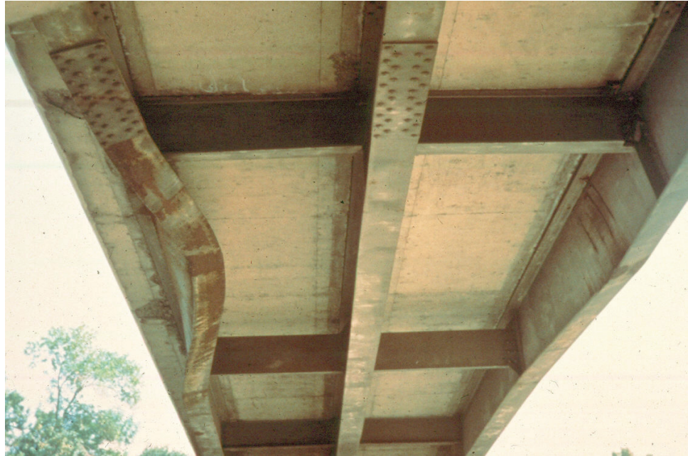
Figure 8.2.24 Collision Damage on a Fabricated Multi-girder Bridge
