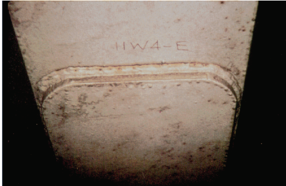
Figure 8.1.32 Part-Through Crack Growth at Cover Plate Welded to Flange
