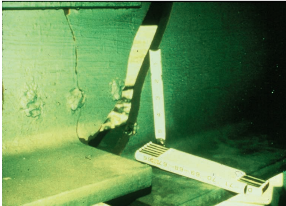
Figure 8.1.23 Crack Resulting from Plug Welded Holes
