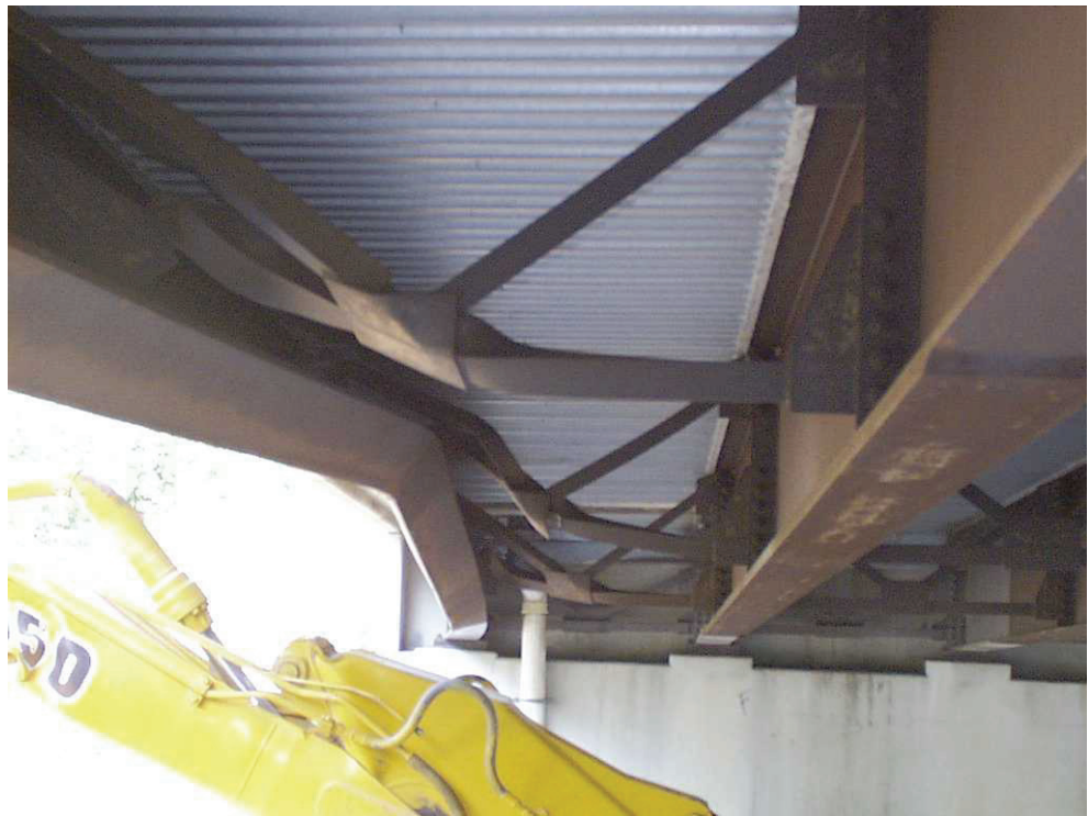
Figure 8.1.28 Severe Collision Damage on a Fascia Girder
