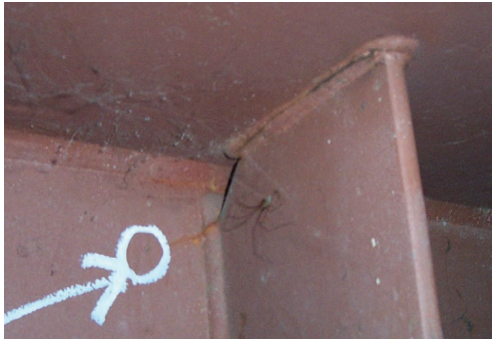
Figure 8.2.28 Web Crack due to Out-of-plane Distortion at Top Flange
