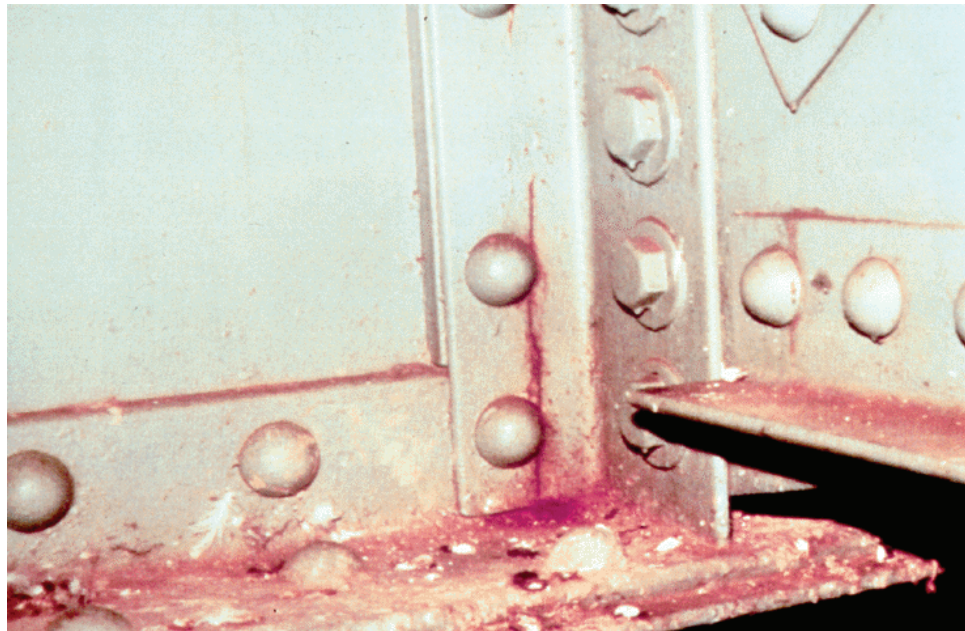
Figure 8.1.49 Cracked Stringer to Floorbeam Connection Angle
