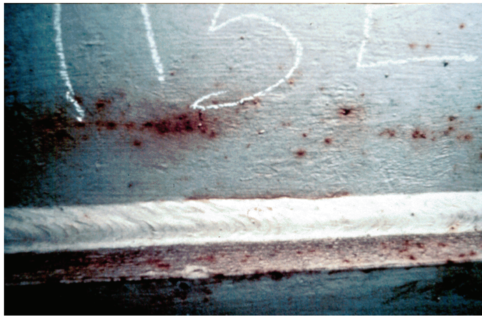
Figure 8.1.31 Part-Through Crack at a Cover Plated Flange
