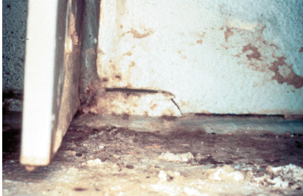
Figure 8.1.40 Through-Crack Ready to Propagate into the Flange
