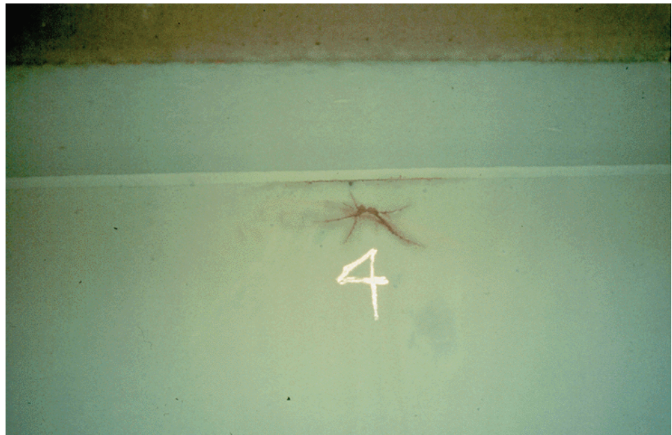
Figure 8.1.39 Through Crack in the Web
