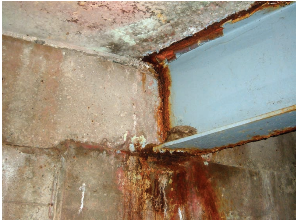
Figure 8.2.16 Corroded Shear Zone on a Rolled Multi-beam Bridge
